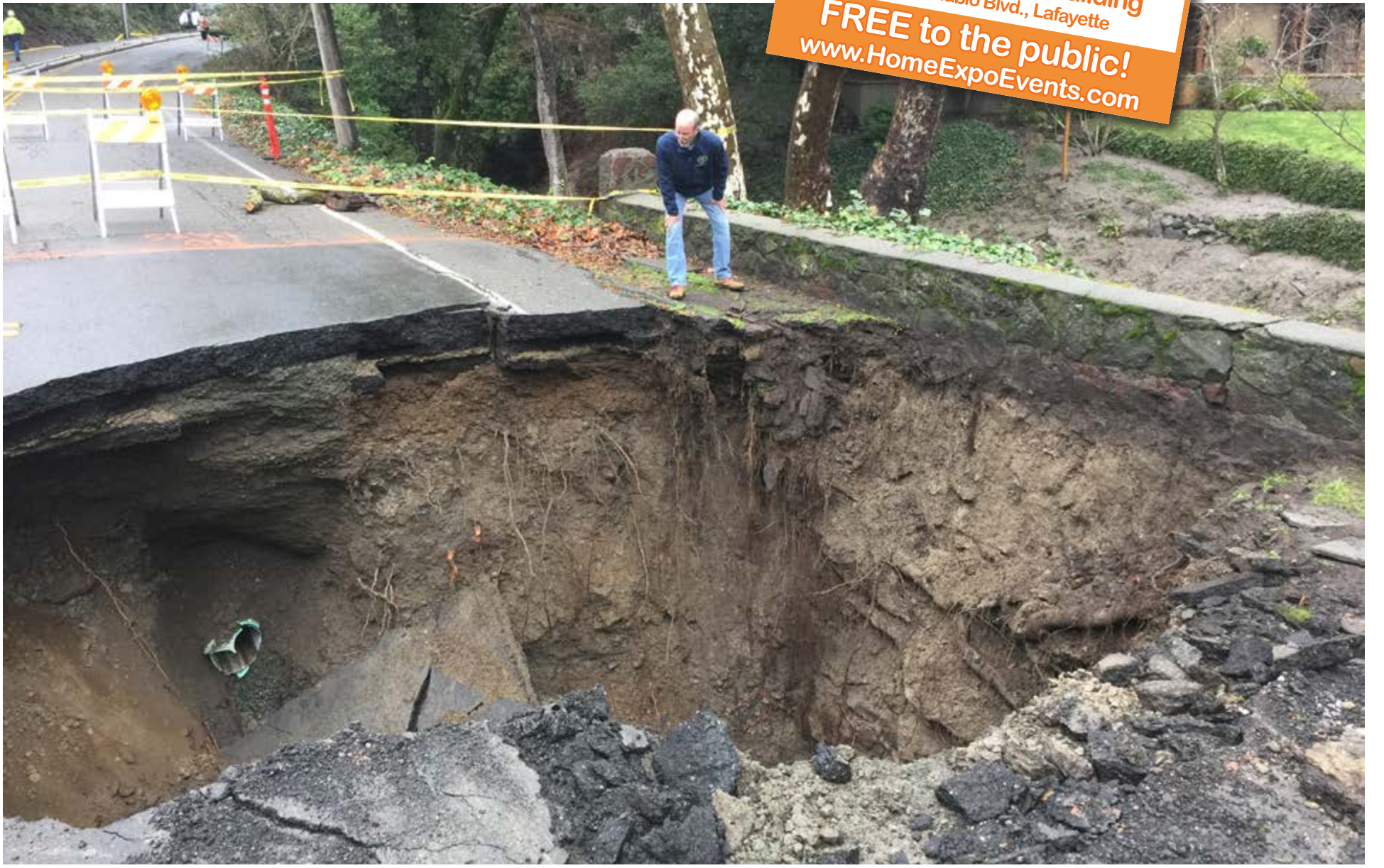
State Senator and Orinda resident Steve Glazer inspects the sinkhole on Miner Road.
